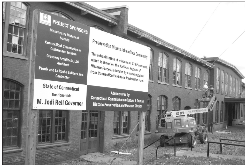
One by one, the windows at the History Center are being restored. We thank all the volunteers who have worked on this project, and all the donors who have given a total of $27,645.00 to preserve the windows of this historic building through the "No Pane, No Gain" fund drive.
