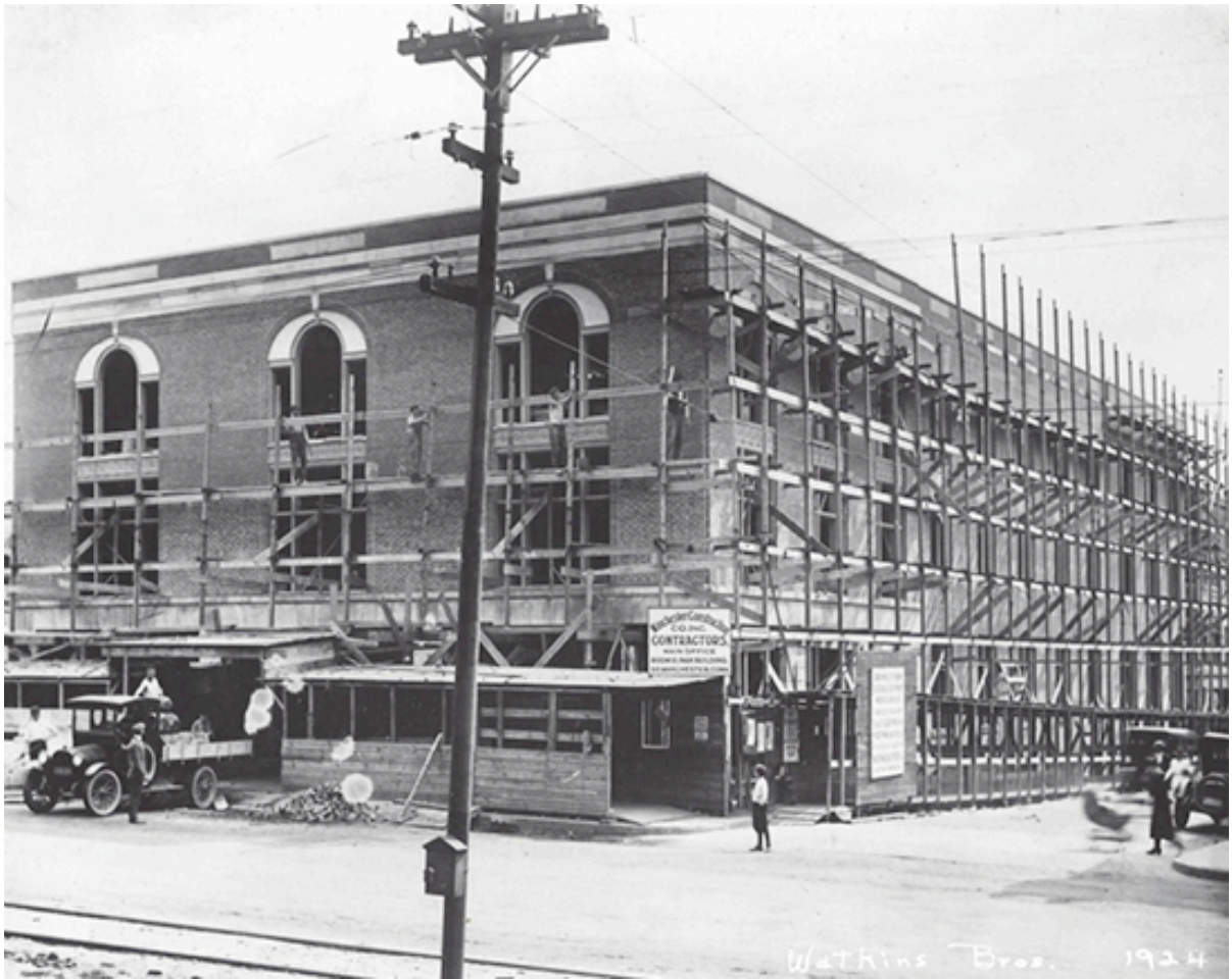
Watkins Brothers block while under construction, circa 1920. The grand opening would occur on November 12, 1920.
